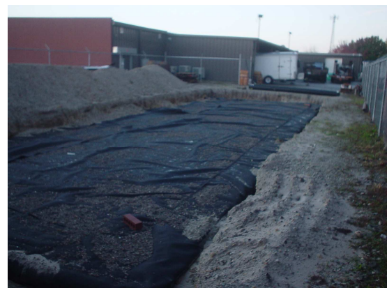
Underground infiltration system
